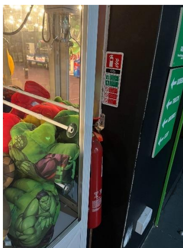
CO2 extinguisher (arcade area)
