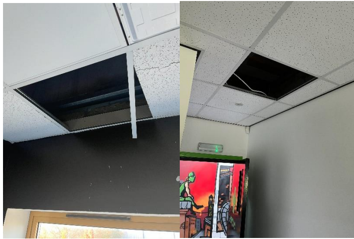
Missing ceiling tiles located in staff room and first aid room
