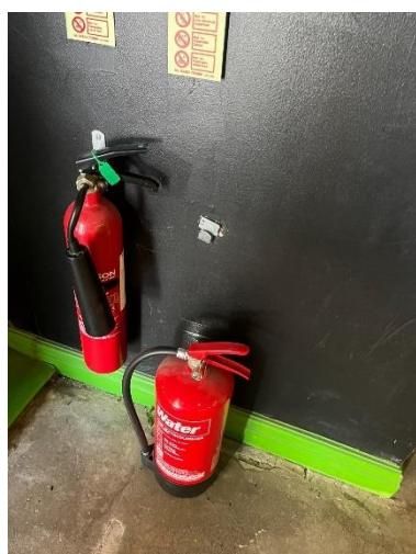
Extinguisher wall bracket
